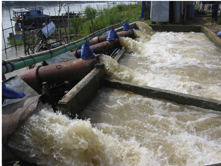
FIGURE 10.3 Pump station for Vietnamese catfish farm.
