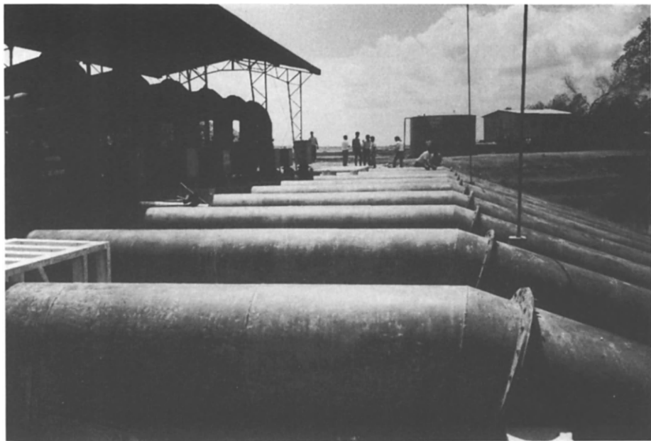
Figure 4. A large, primary pump station on a semi-intensive shrimp farm of more than 800 ha in Ecuador. Ten diesel driven pumps delivered water from the source estuary to the reservoir canal.
